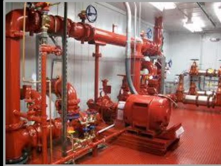
ELECTRIC FIRE PUMP
