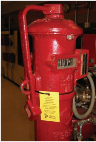
Post indicator valve closed
