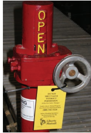
Post indicator valve open
